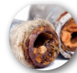
Internal Pipe Corrosion
