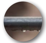
External Pipe Sweating
